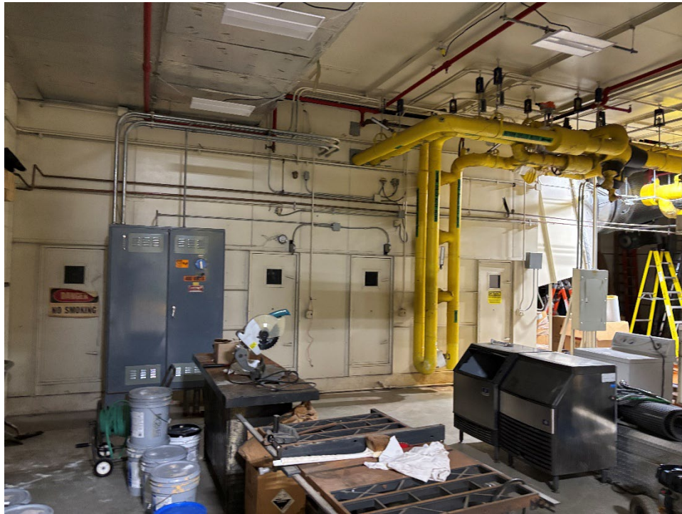
View looking West towards AHU inside Mechanical Room
