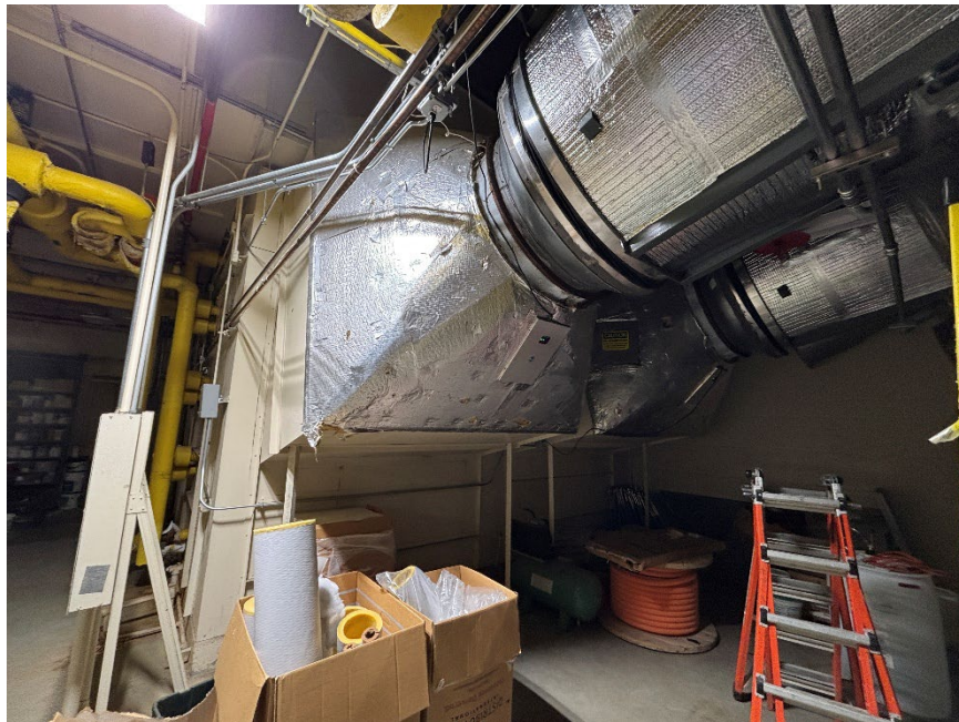
North end of the AHU
