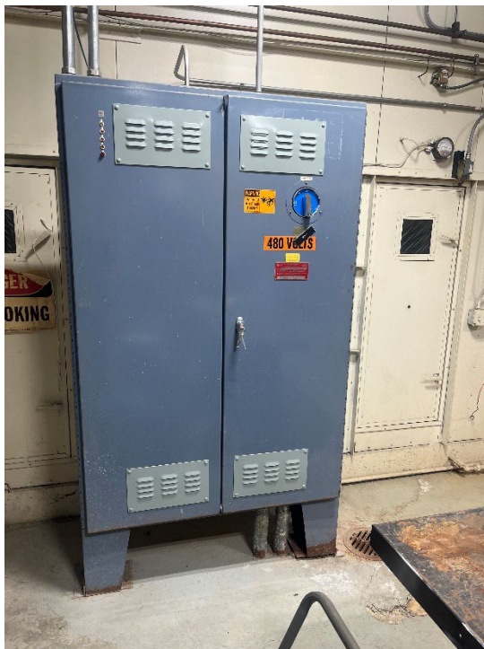
Existing Electrical Panel
